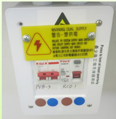
Fault Current Protection
