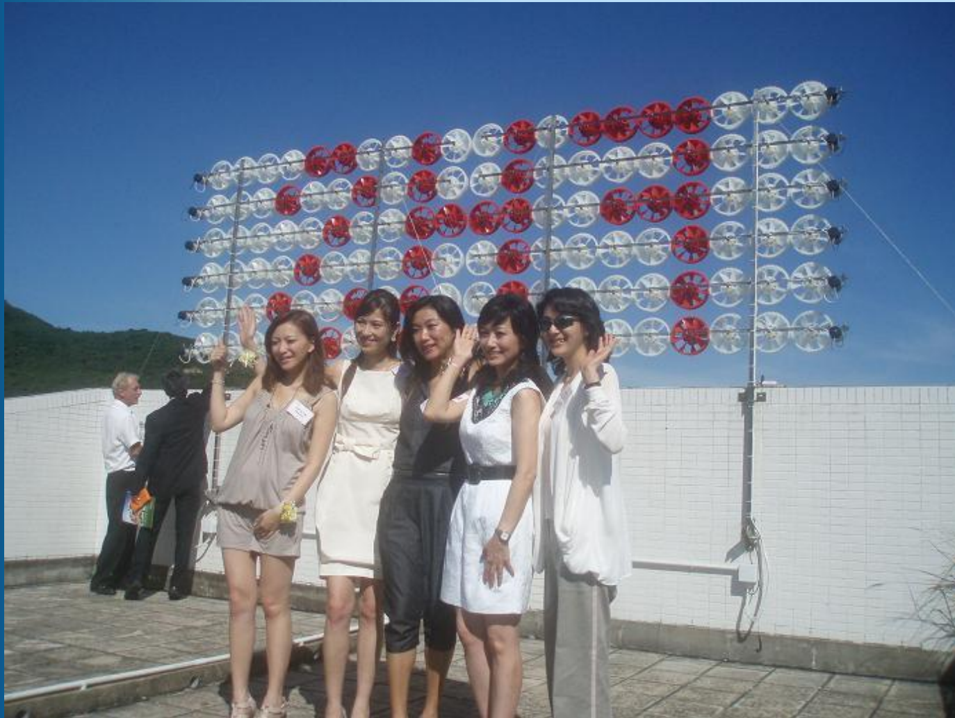
Fu Hong Society - Aberdeen 扶康會 – 香港仔 Consists 2 x 120 micro turbines Installed in August 2010
